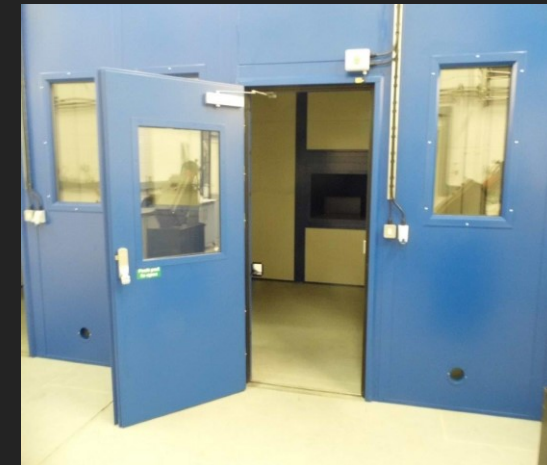
Acoustic Doors with closers and drop seals to complete the installation
