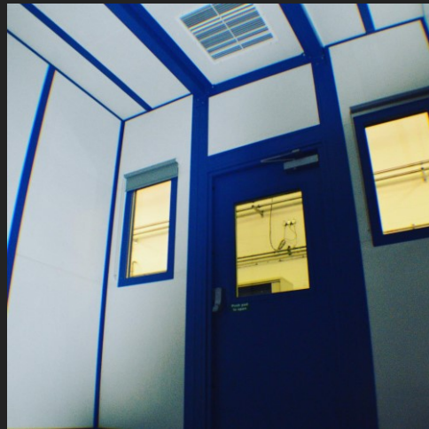
Inside the enclosure. Showing the internal surfaces powder coated in white to compliment the exterior colour
